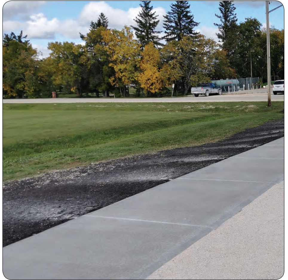
EXPRESS PHOTOS SUPPLIED BY THE RM OF WEST INTERLAKE The 54-metre sidewalk connects the STARS landing area to the EM Crowe Memorial Hospital across the street.
