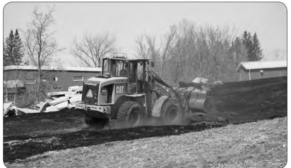
Crews plow up the burnt area near the RM's public works storage site.
