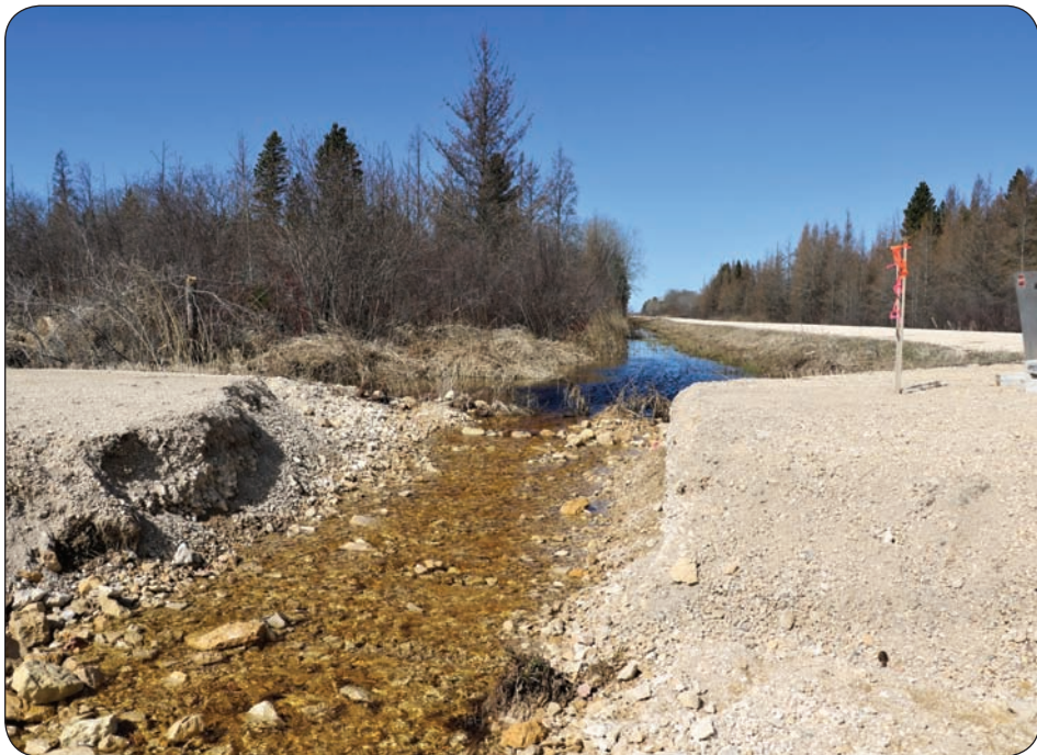
Runoff took out Road 9E at 124 NE in the RM Armstrong. Photo taken April 28.
