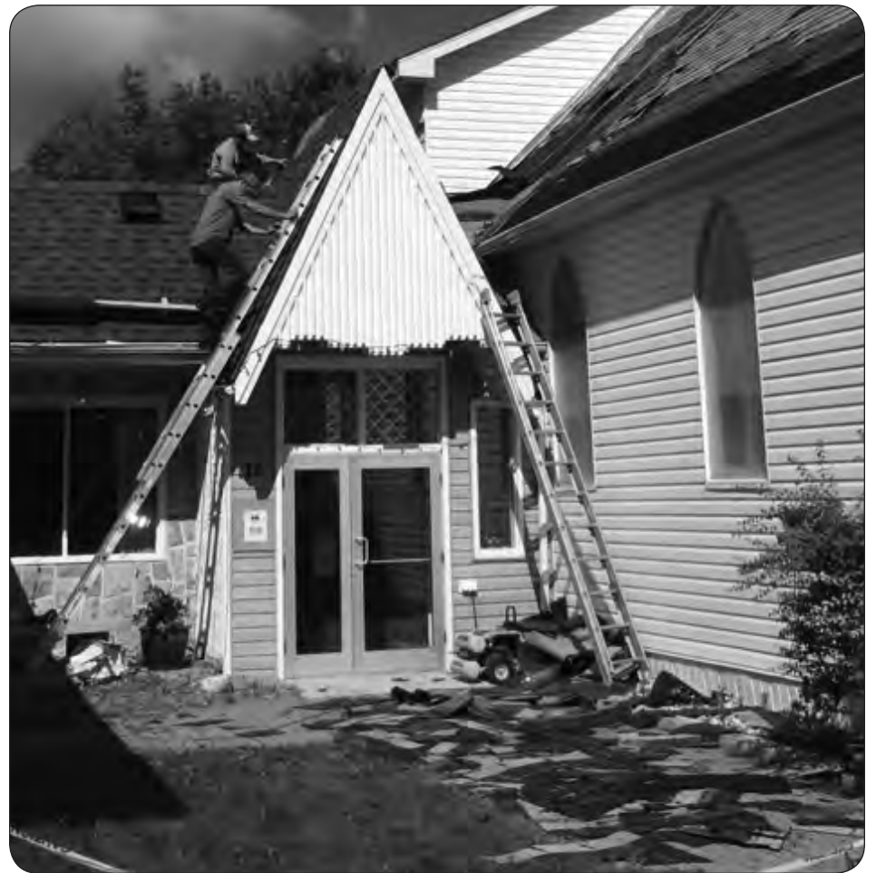
EXPRESS PHOTO SUBMITTED BY ALVIN GORANSON Workers from Wall Brothers Construction took two weeks to completely redo the many roofs of the Lundar Lutheran Church.
