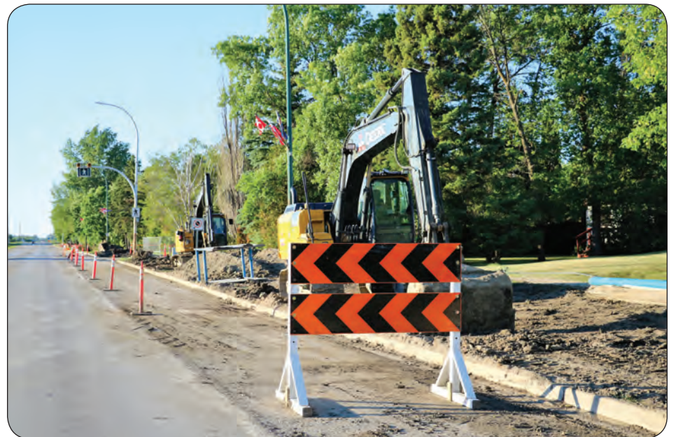
EXPRESS PHOTOS BY PATRICIA BARRETT Upgrades to water lines along Highway 9 continues.
